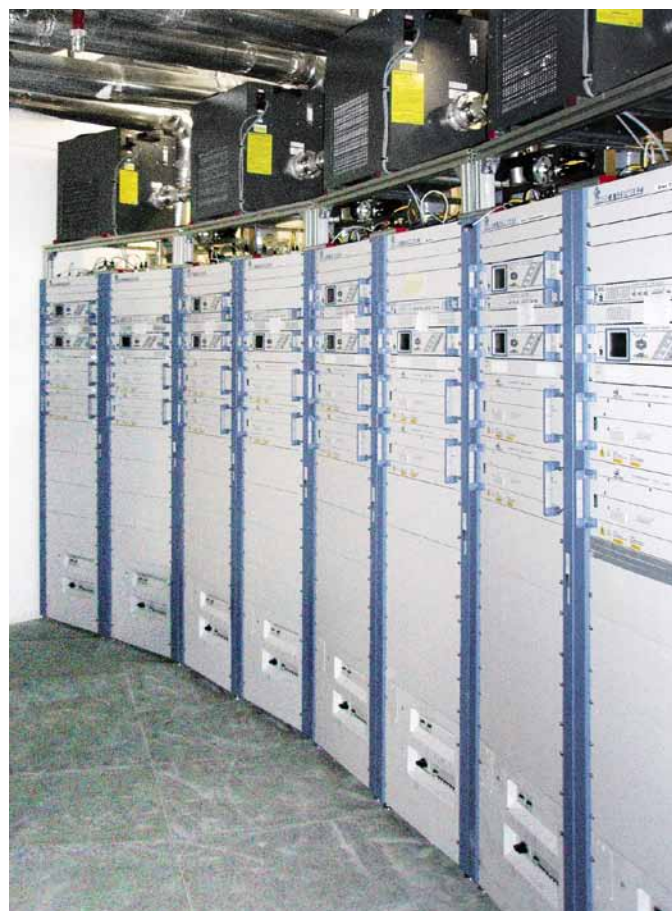
Fig. 2 Some of the R&S®NR8205E VHF FM transmitters that were successfully installed on the 31st floor.
